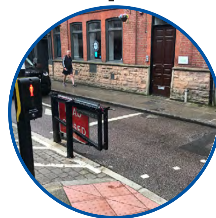
Gate for road closure
